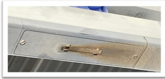
Static Sensor Operated with Contaminated Purge Air
